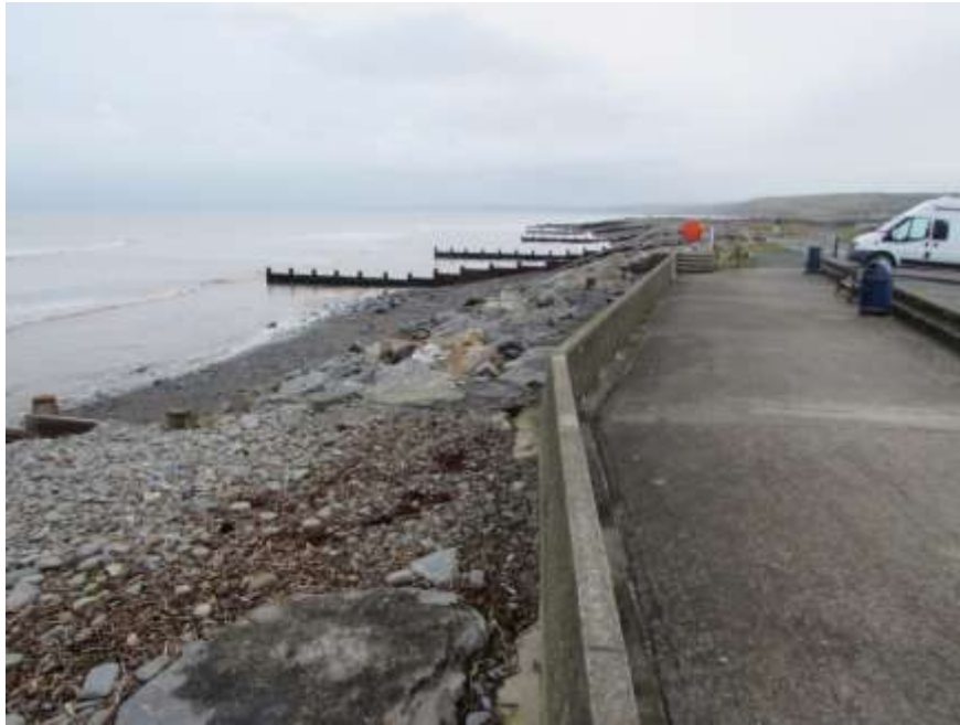
Figure 50 Sediment starved shingle beach down-drift of Aberaeron harbour entrance piers
