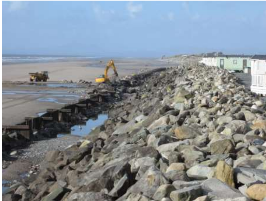
Figure 51 Use of rock armour and sheet piling to protect a caravan park and Cambrian Coast Railway, on a former shingle ridge, north of Llanaber, Gwynedd
