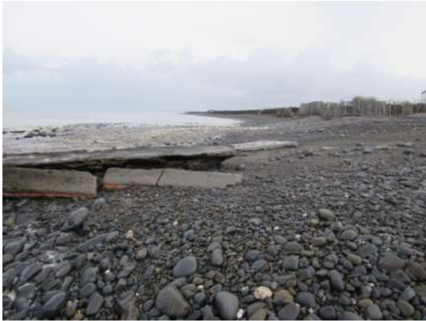
Figure 58 Degraded concrete groyne built to limit shingle drift towards the stream outlet shown in Figure 57
