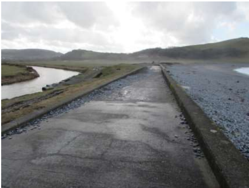
Figure 56 Concrete sea wall and promenade / roadway separating the River Ystwyth from the beach at Tanybwllch, south of Aberystwyth
