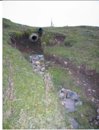
Road drain that likely contributes to spring flows during periods of high rainfall (upper part of site)
