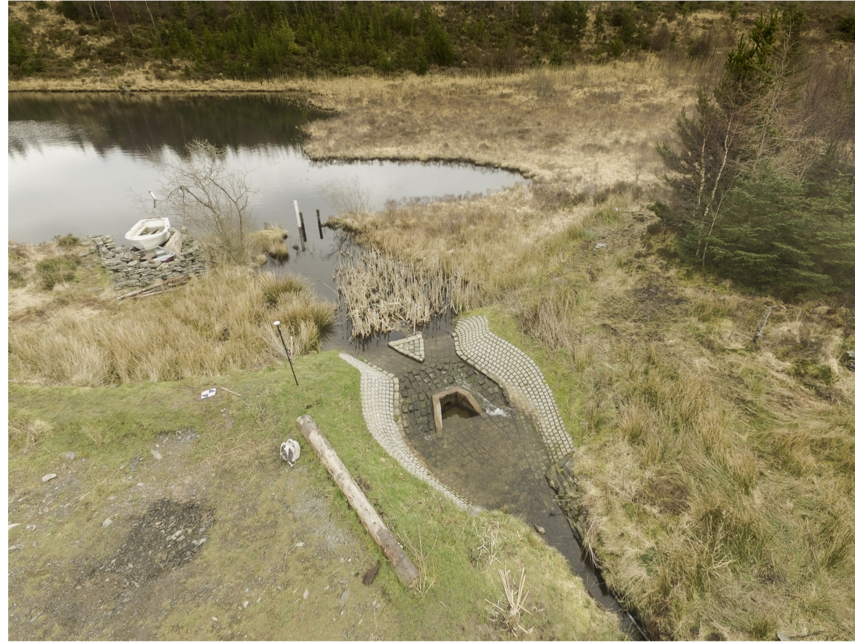
Awyrlun o'r gronfa a'r argae presennol Aerial photograph of reservoir and existing dam
